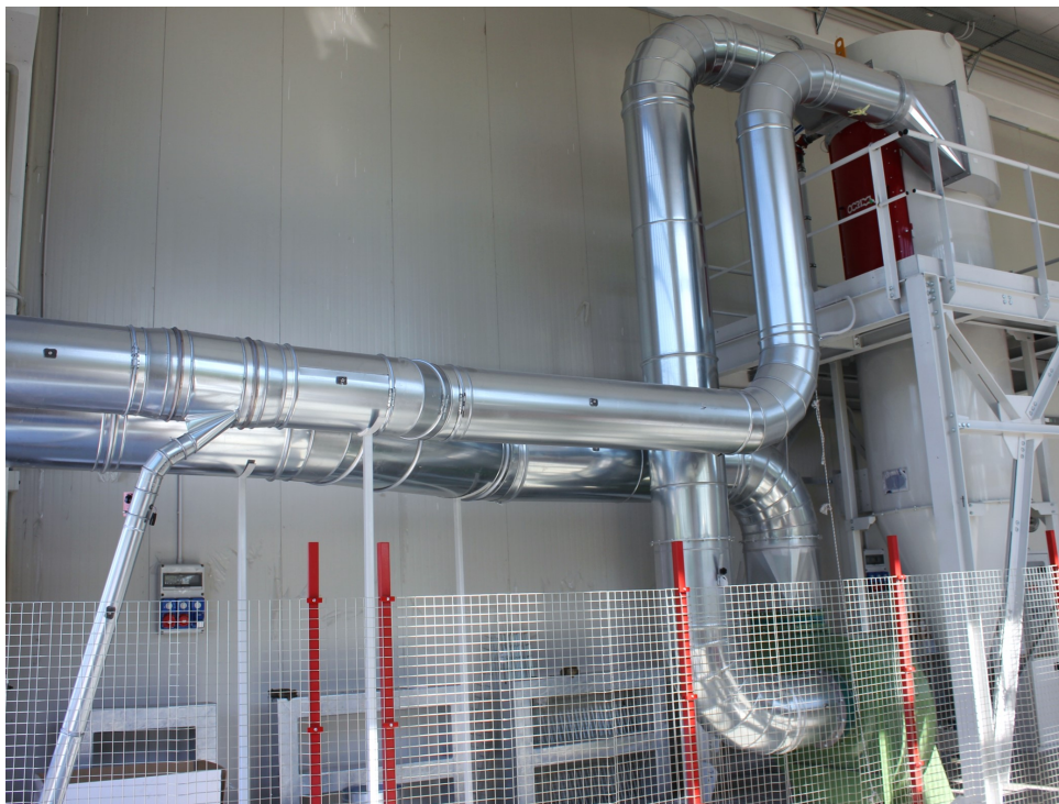
Figure 4.2: Pilot plant with a cyclonic bag separator installed at the University of Parma, Italy.
