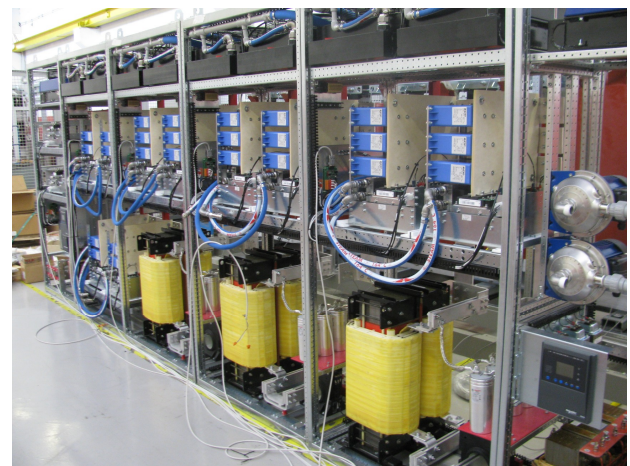
Fig. 23. Picture of one of the 2 MVA converters.
