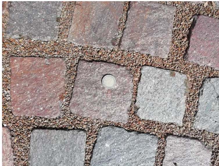
318 319 Figure 8 - Too wide joint width in a stone cube pavement
