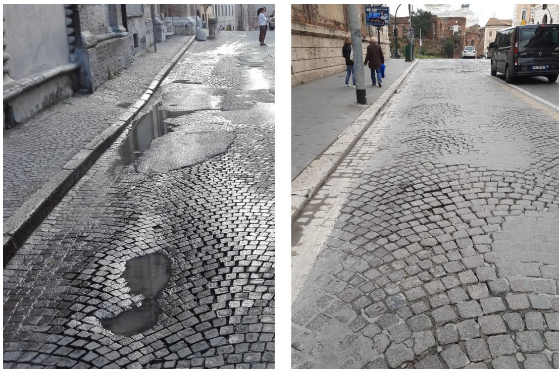
463 464 Figure 12 – Stone pavements affected by faulting, punching, horizontal creep and asphalt 465 patching
