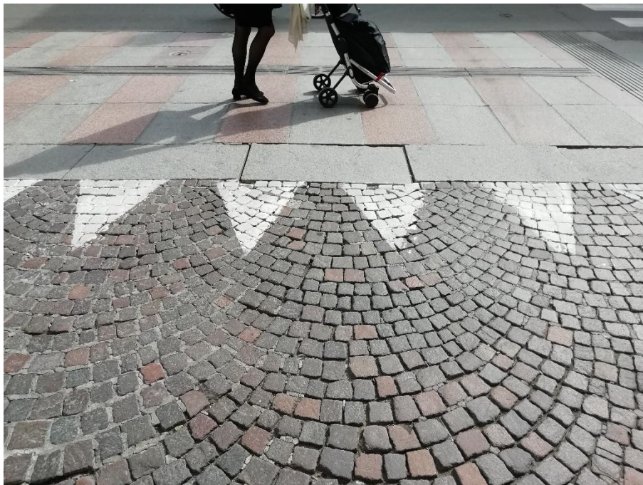
437 438 Figure 11 - Stone pavement defects at stop/start line
