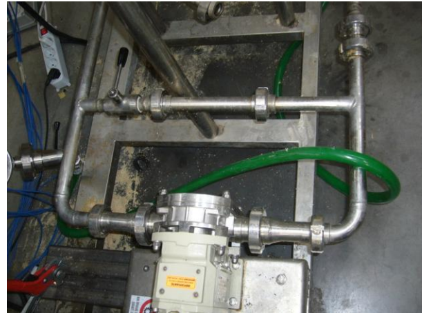
Figure 3.7: The recirculation circuit.
