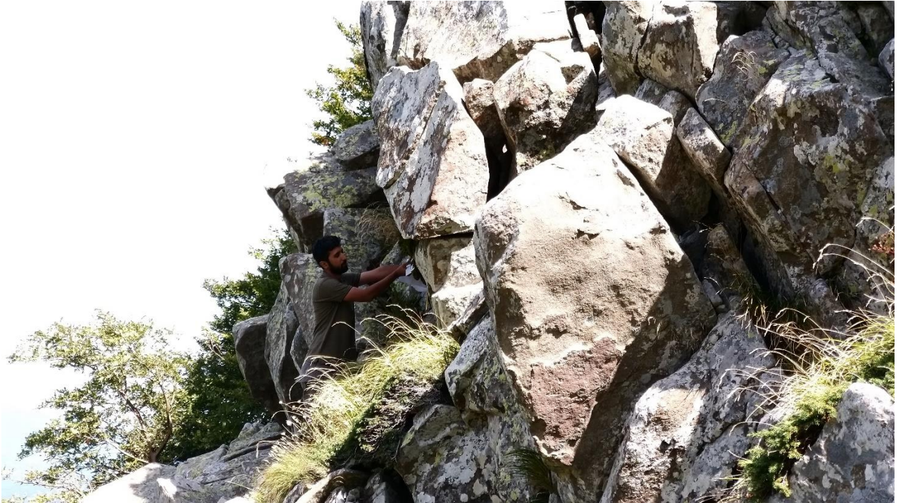
Figure 3.6: Fractured Macigno Sandstone rock near Alpe di Succiso. A person (~1.80 m tall) is shown for scale.
