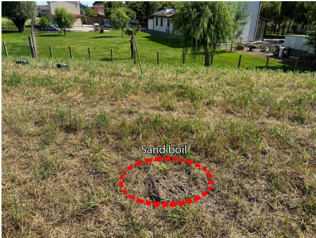
Figure 4.18 - Sand boil related to water infiltration.
