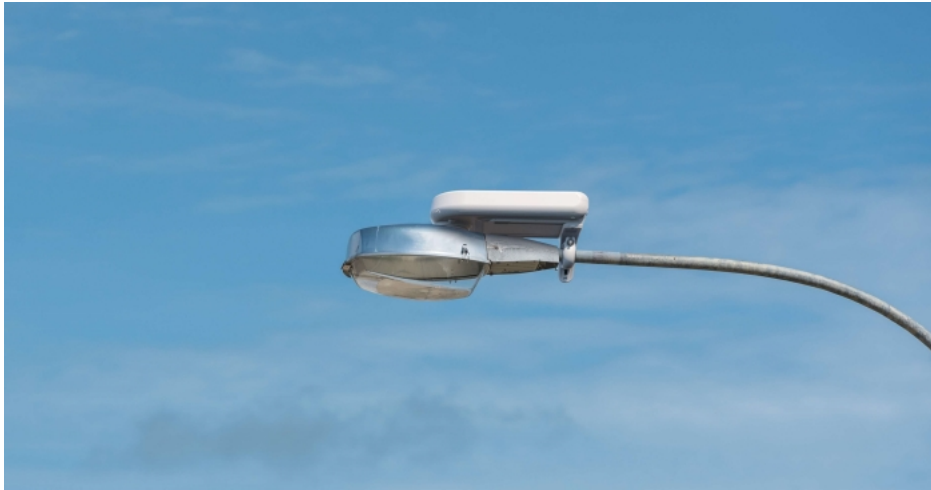
Figure 4.9: 5G small cell (provided by Ericsson [1]) installed on a street light.
