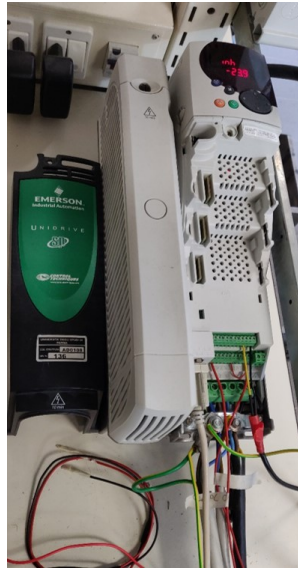
Figure 1.22: Commercial motor test bench inverter, Emerson UNIDRIVE
