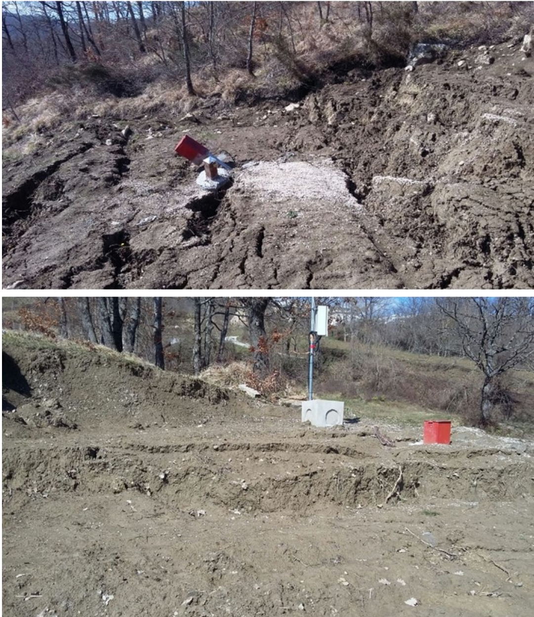
Figure 58. Area surrounding Vertical Array DT0014 as seen during the on-site inspection (Segalini et al., 2019a)
