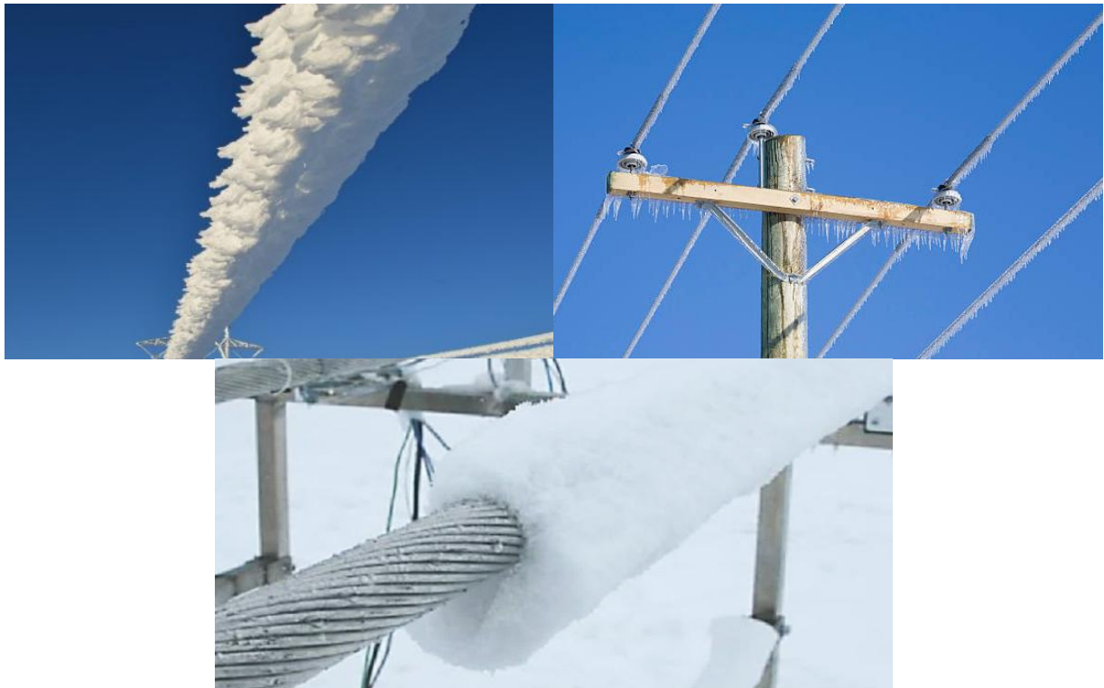
Fig. 10 Example of sleeves grown on conductor cables. Clockwise: rime ice (top left), glaze ice (top right) and wet snow (bottom).
