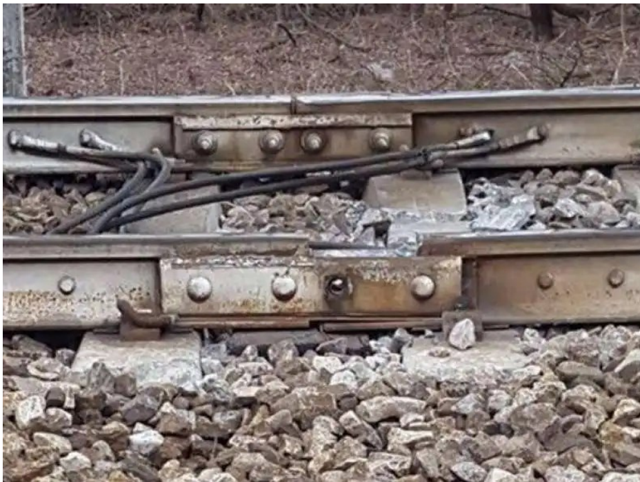
Figure 29. IRJ collapsed: a bolt is missing, and material has completely detached from the rail head
