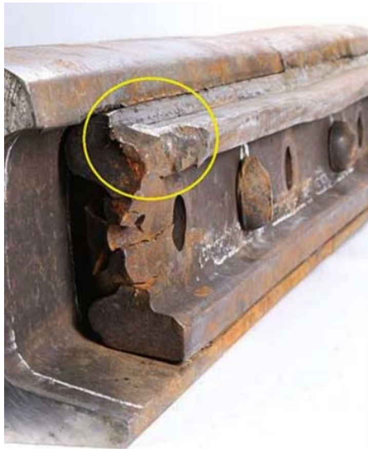
Figure 21. Loss of IRJ bolts
