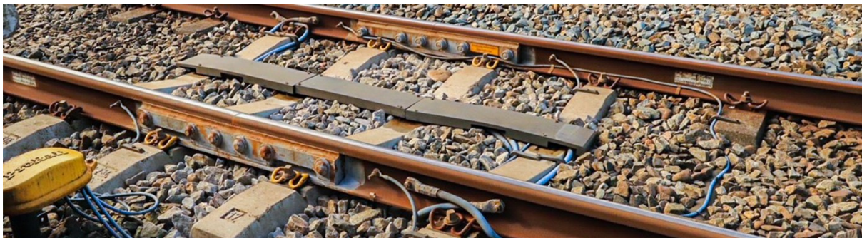
Figure 23. Evident instability of the ballast due to IRJ
