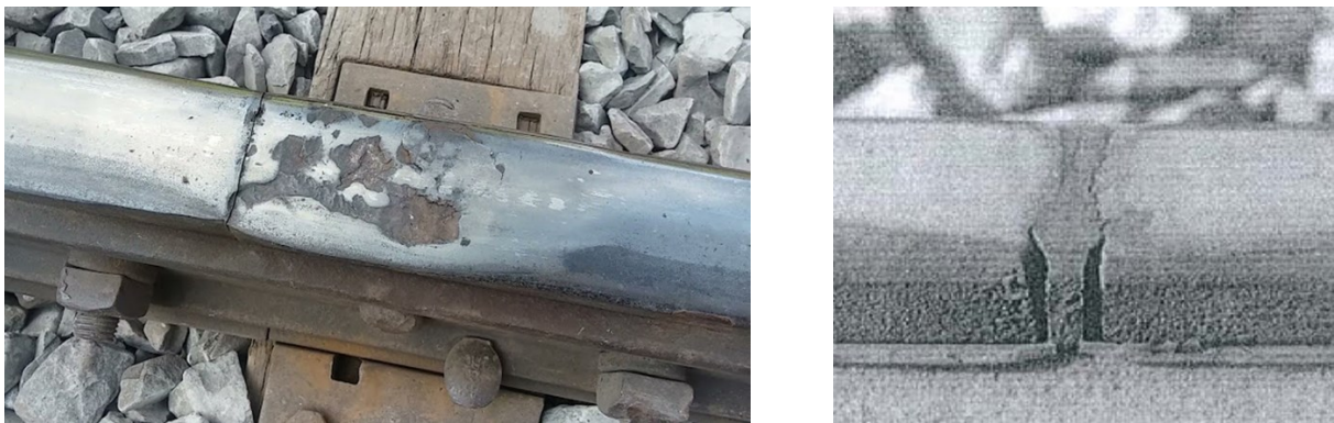
Figure 22. Battered rail ends and delaminated end post
