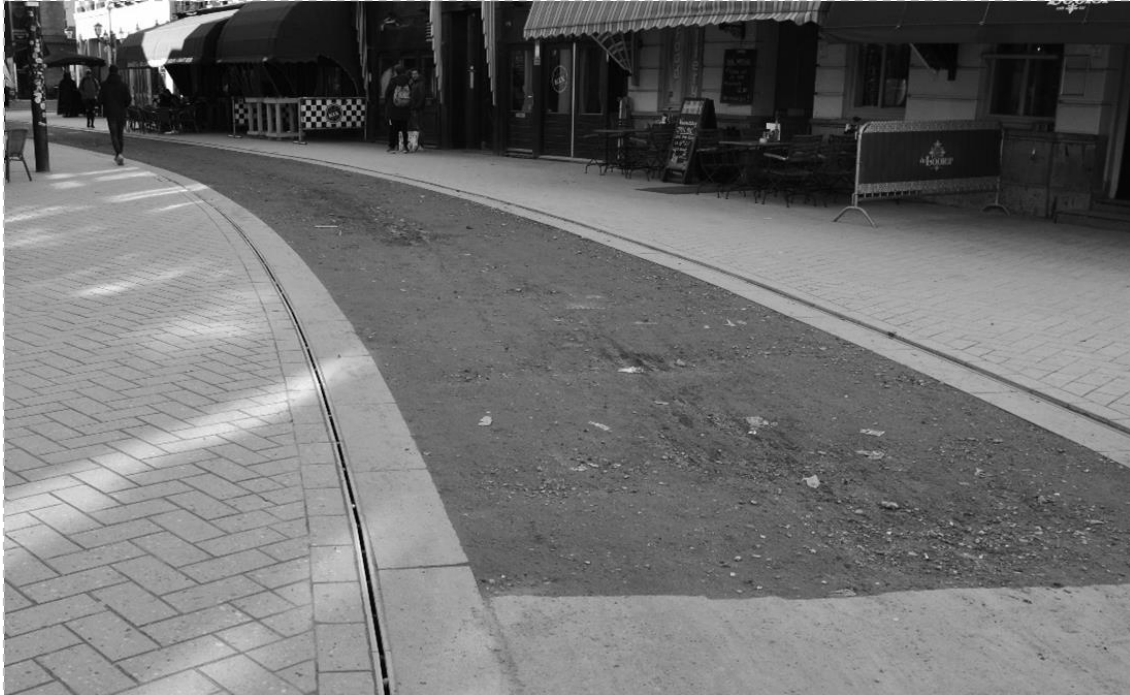
Figure I.18 | Construction site of a street renovation in Eindhoven, the Netherlands. Source: photo taken by the author (2023).
