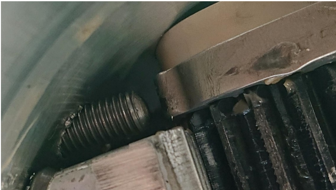
Figure 66. Check of the components of the cam – M8 stud bolts connection after testing at 10.5 barg.
