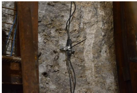
Fig. 3.15: Tunnel Link sensor installed on site
