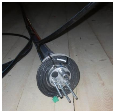
Fig. 3.16: Rad Array installed together with a Multi-Point Rod Extensometer
