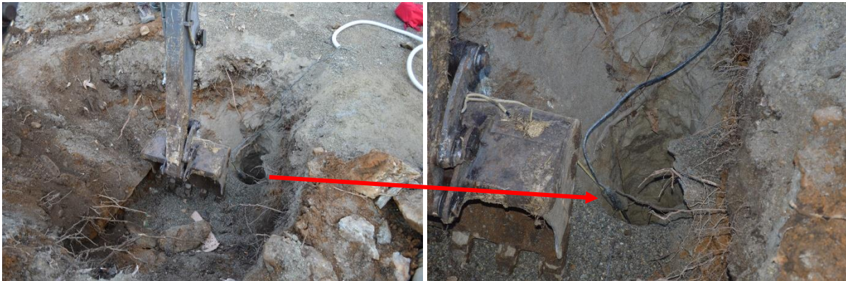
Fig. 3.18: Recovering of the array after an incorrect installation procedure
