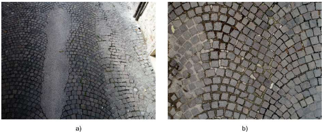
179 Figure 3 – Distresses detected on the stone pavement during the survey.
