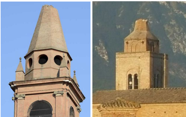
Figure 2. Damages to belfries spires in the 2012 Emilia earthquake (left) and in the 2016 Central Italy earthquake (right).
