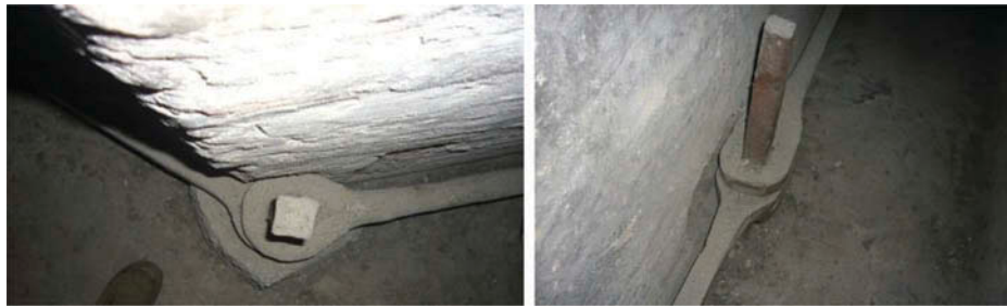
Figure 22. Pictures of the first iron chains inserted by Vasari, in 1570, in the corridor between the two shells.
