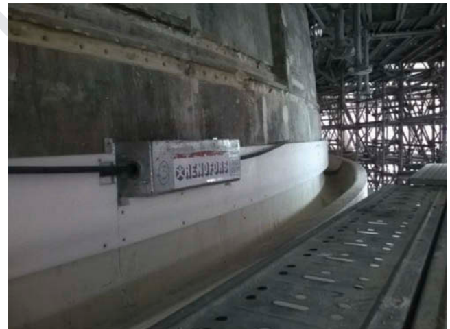
Figure 16. The new iron hoopings, realized by two pre-tensioned high resistance cables, recently added around the French Pantheon dome.
