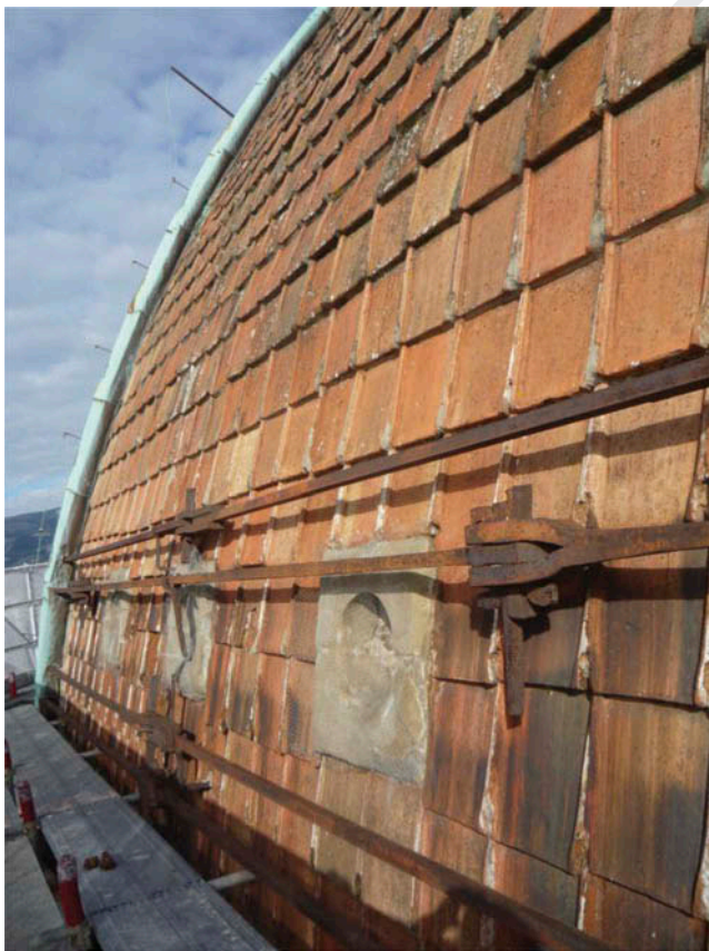
Figure 23. Picture of the iron chains at the extrados of the dome, which are free from rib to rib.
